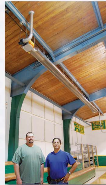
Kevin Neese, Director of Maintenance and Facilities for the Moffat School, credits Anthony Garcia, Project Manager for Vendola Plumbing and Heating for the Solaronics heating system specification and installation.
