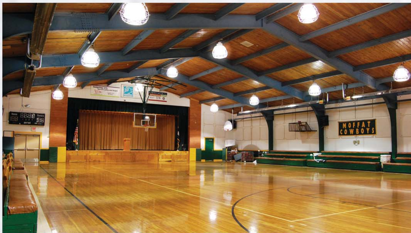
In addition to sports, the Moffat School Gymnasium hosts plays, concerts, community events and local government meetings. The Solaronics heaters are appreciated as much for their silent operation as for the comfort heating and energy savings they provide.
